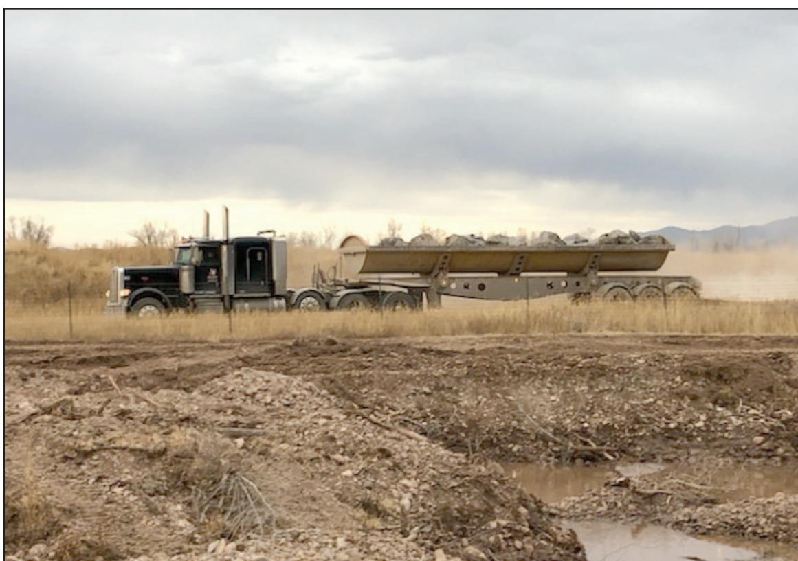
Rock donated by Itafos Conda Phosphate Operations in Conda, ID is hauled to the project site for construction. [Photo: SVCD]
